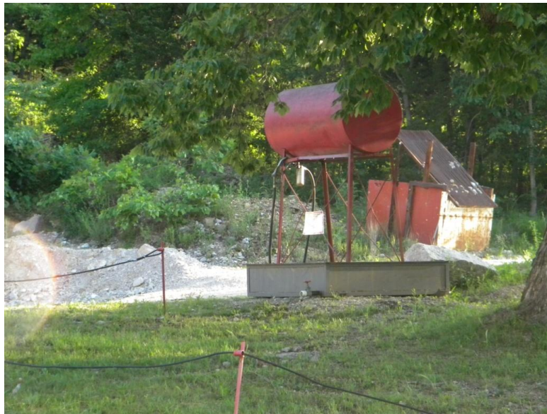
Figure 5.3. Diesel Fuel Tank at S&T's Experimental Mine
