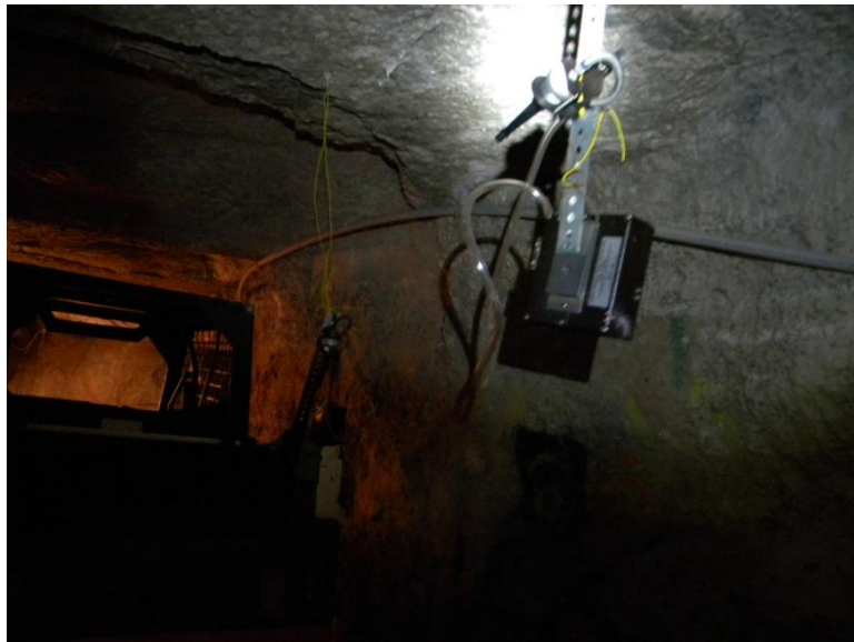
Figure 5.7. Installation of the Sampling Train at the Back of the Entry
