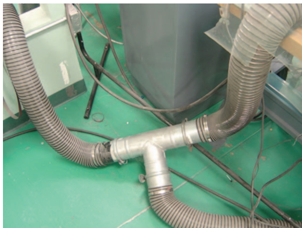
FIGURE 3. Local exhaust ventilation flexible ductwork connected with a T-junction at the box polish station with (photo by NIOSH).
