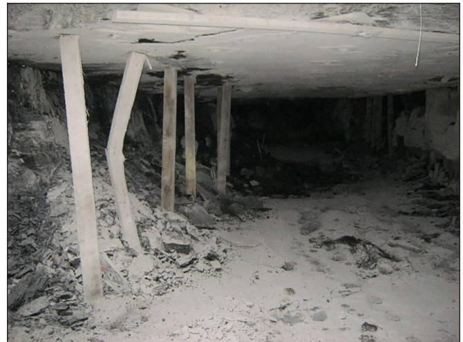
Figure 4. Photo taken on Dec. 3rd, 2014, depicting rib sloughage with a broken post indicating additional convergence
