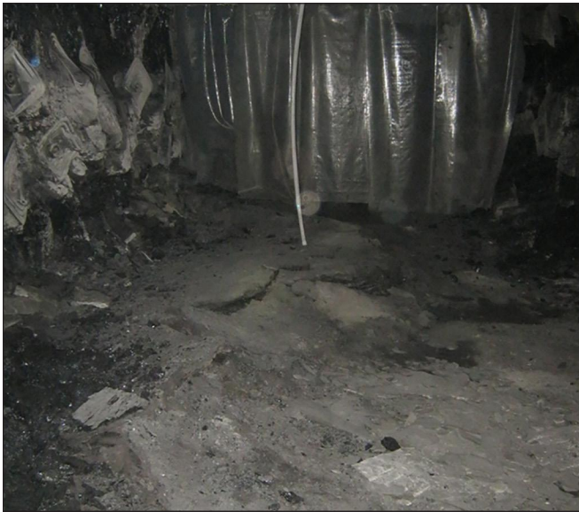
Figure 5. Area where 15 in. of floor heave was measured showing bent pogo stick
