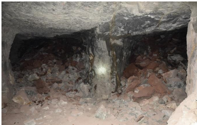
Figure 3: Two near-vertical, large iron-stained joints in a pillar nearby the collapsed area.
