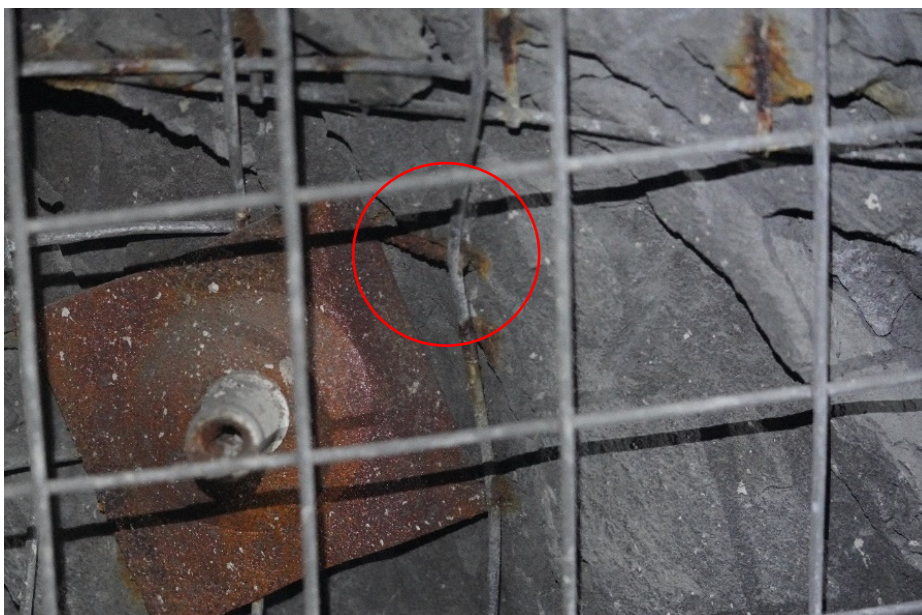
Figure 1 Observed galvanic corrosion in partner mine where metal ground support contacts the graphite-like rock
