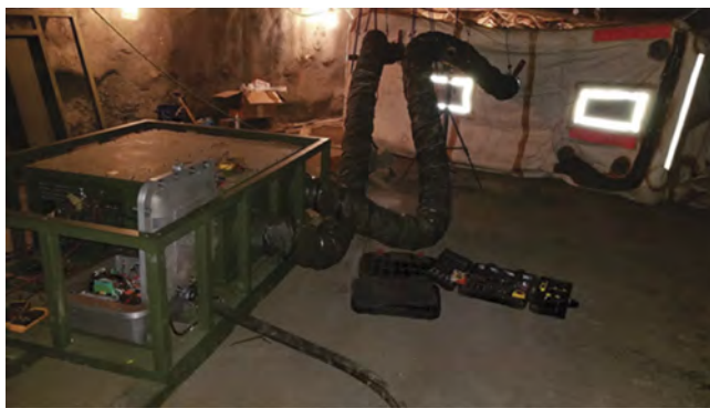
Figure 2. Picture of a BPAC connected to a portable tent-type RA using flexible duct.
