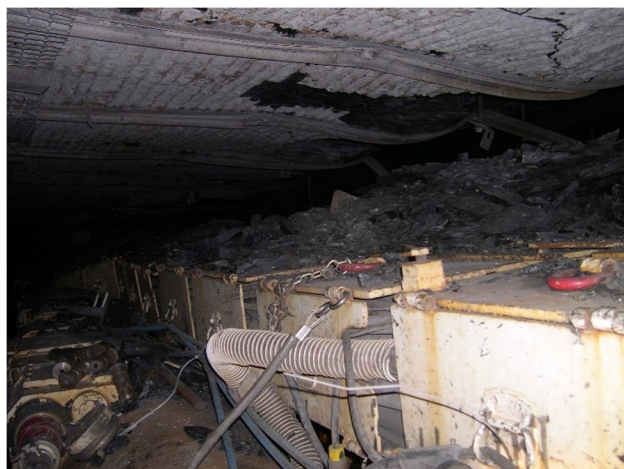
Fig. 4 Roof cutter developed at the belt entry corner on the panel side
