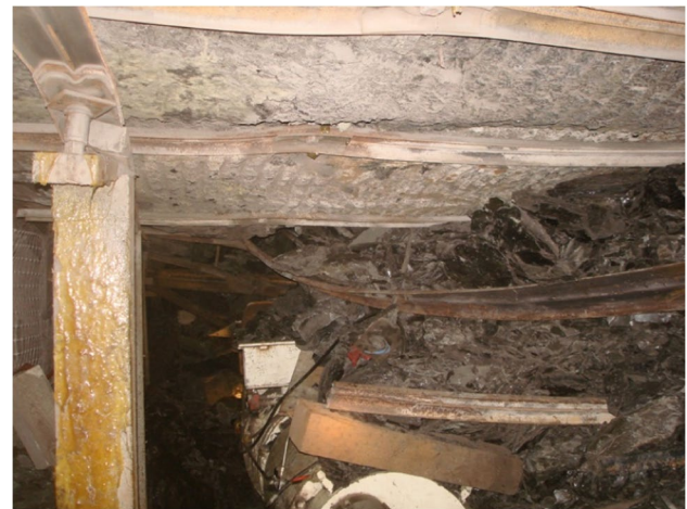
Fig. 2 Roof fall near the face in the belt entry
