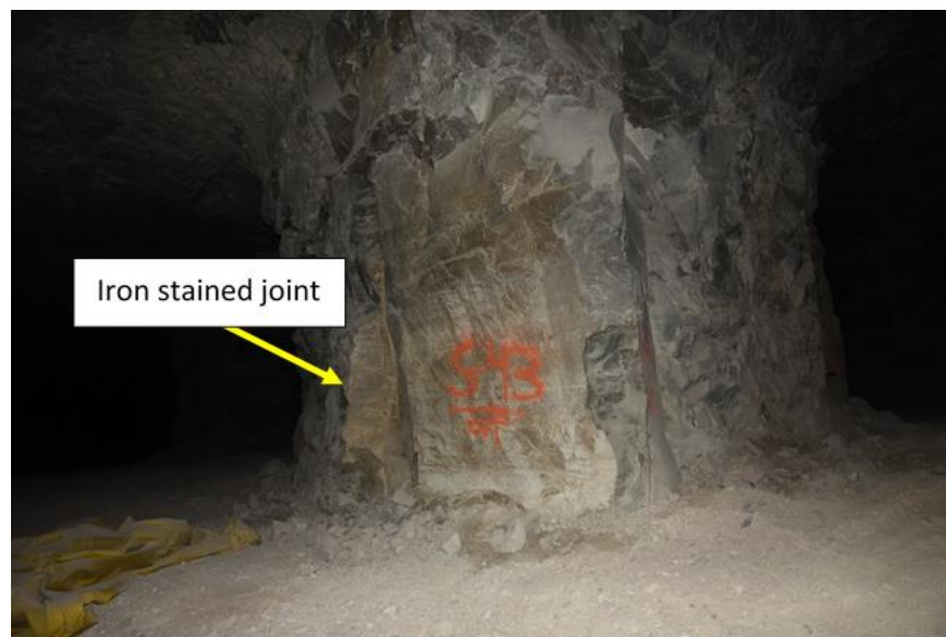
Figure 6. Iron stained joint in a pillar on the edge of the collapse area.
