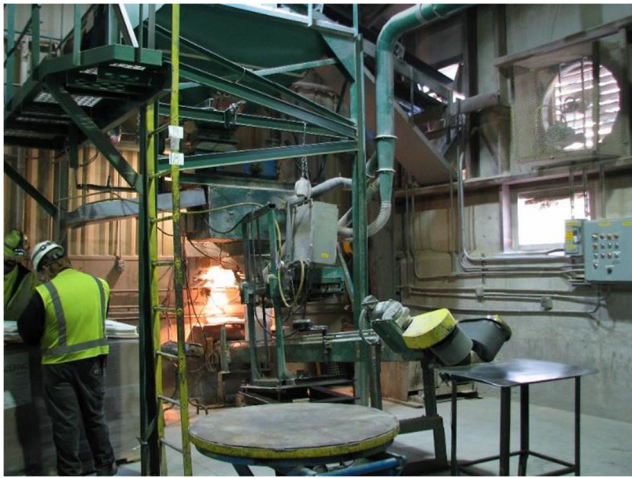
Fig. 8 Manual bagging machine and wall ventilation fan on the top right corner
