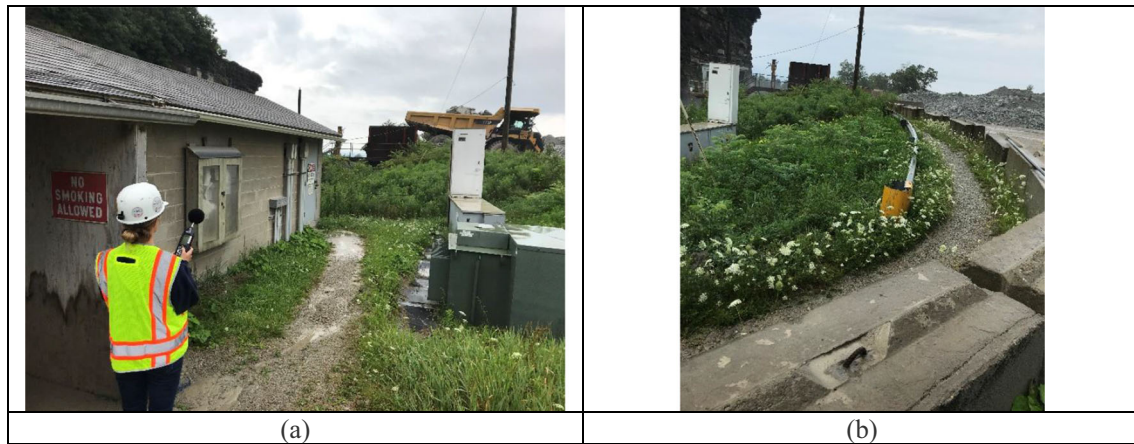
Fig. 27 Outside area near the control room of the primary crusher
