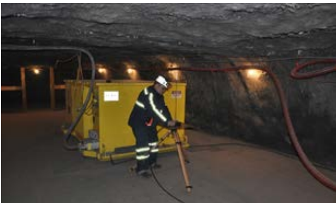
Figure 3. NIOSH Experimental Mine Power Center.
