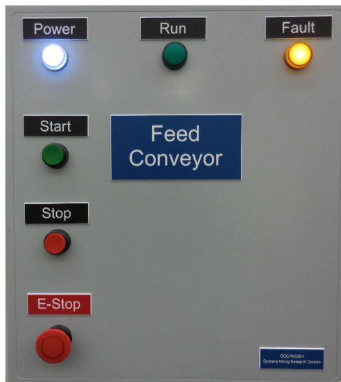
Fig. 8 Motor controller with Power and Fault indicators illuminated
