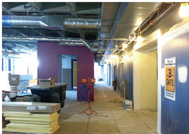
Housekeeping issues bedevil many jobsites; B-SAFE helped prevent slips, trips and falls. “The trades were working together with the B-SAFE program, and other trades were watching out for everyone else. Normally they would never do that, but now I see talking amongst the trades – this came from the program.” (B-SAFE site employee)
