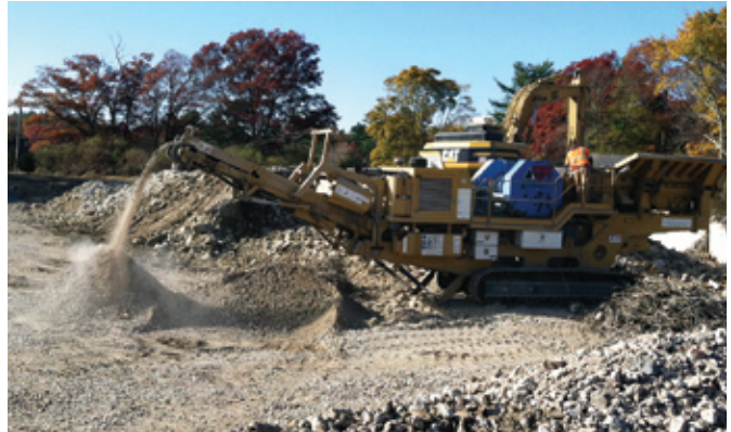
Rock crushing (above) creates high levels of silica exposure, but researchers found misting equipment provided valuable protection to workers.
