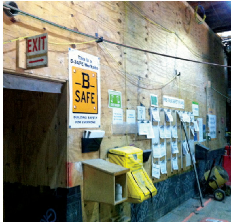
B-SAFE sign adjacent to the pre-task planning board serves as a reminder. Site managers report an increase in safety awareness and teamwork.
