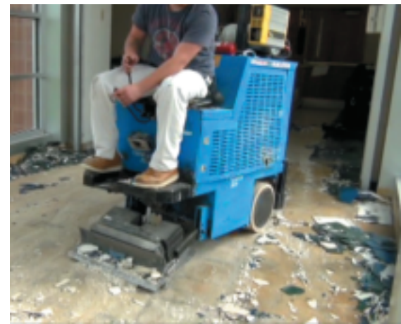
Breaking tile, not backs, can be done with a ride-on floor scraper, the “Terminator.”
