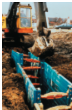
Gallegos' search ended on eLCOSH with this photo showing a poorly installed shield that would not restrict hazardous lateral movement.
