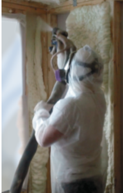
Redlich's team wants to know ... how safe is spray foam insulation for the workers using it?
