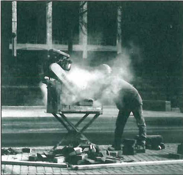
Worker exposed to dust while cutting paving bricks.
