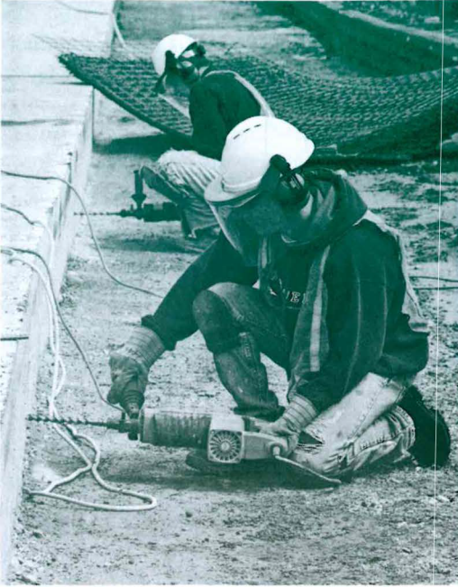
Figure 19-6. Example of worker using multiple forms of personal protective equipment, including hard hat, face shield, hearing protection, work gloves, knee pads, and work boots. (Photo Courtesy of Mine Safety Appliance Company.)
