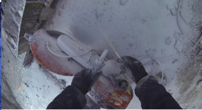
Figure 40. Indoor Athletic Facility: Water Tank Hose Disconnecting Mid-Cut
