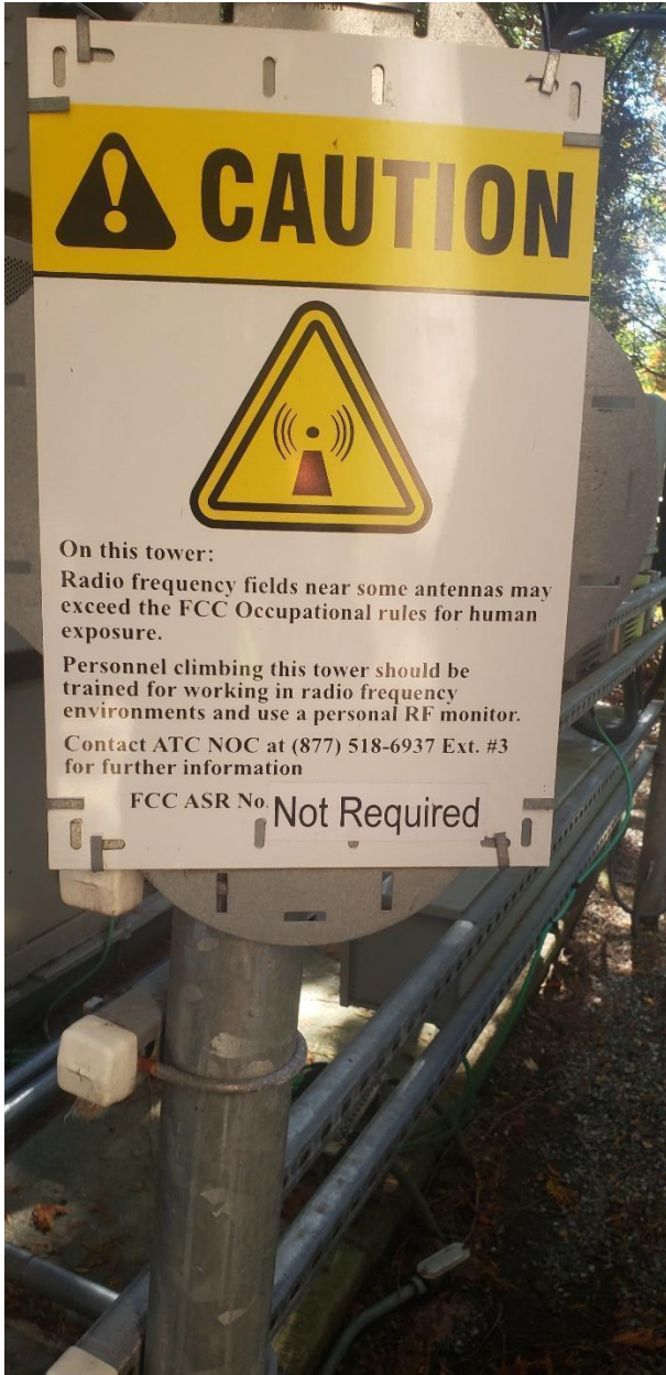
Figure 24. Warning label on base of above shown cell tower
