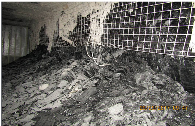
Fig. 1. Extensive rib damage in an underground coal mine in the Western US.
