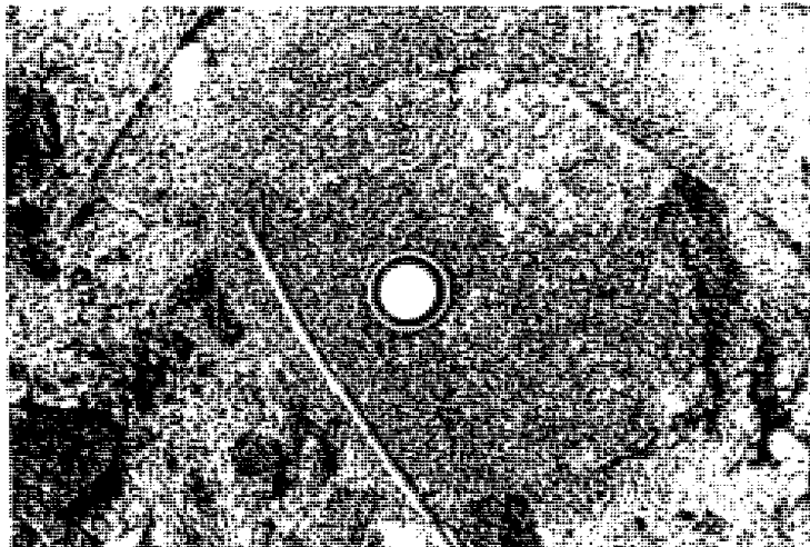
PHOTO B. SLAKING SHALE ON LEFT ABUTMENT REMNANT OF DAM NO. 3. FAR MORE COMMON THAN THE SLAKING MODE ILLUSTRATED ABOVE, HERE THE SHALE SLAKES INTO PUNKY, SOFT FRAGMENTS LESS THAN 1/2 INCH LONG. FOR SCALE, LENS CAP IS 2-3/8 INCHES IN DIAMETER.
