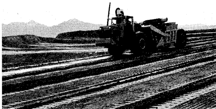
PHOTO C. VIEW SHOWING ELECTRIC SELF-LOADING SCRAPER EXCAVATING COARSEST TAILINGS FOR CONSTRUCTION OF PERIPHERAL EMBANKMENT.
