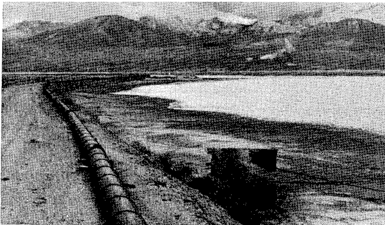
PHOTO C. VIEW OF CEMENT-LINED SPIRALWELD STEEL PIPE USED FOR TAILINGS DISTRIBUTION AT KENNECOTT'S TAILINGS DEPOSIT NEAR SALT LAKE CITY, UTAH.
