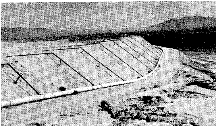
PHOTO C. TRANSITE HEADER PIPE WITH LATERALS USED IN DISTRIBUTING TAILINGS AT THE MISSION UNIT OF THE AMERICAN SMELTING AND REFINING COMPANY, ARIZONA.
