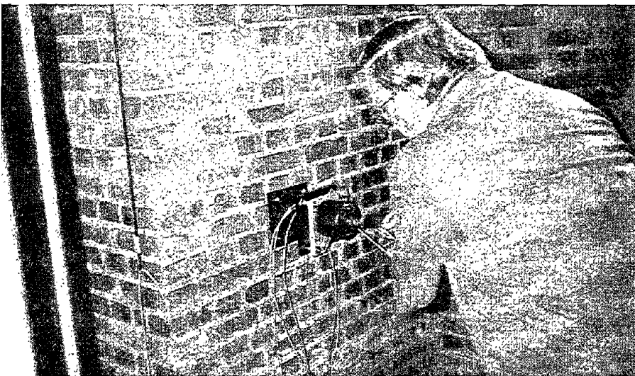
Installing a tiltmeter to measure changes in the tilt of the cathedral towers.
