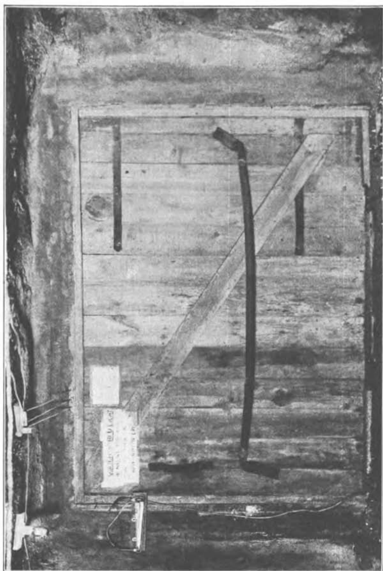
FIGURE 19.—Ventilation door between butt entries
