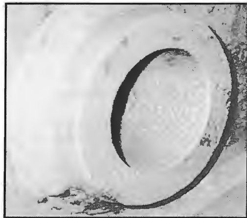
Figure 8.—Corrosion of a lemniscate link clevis.
