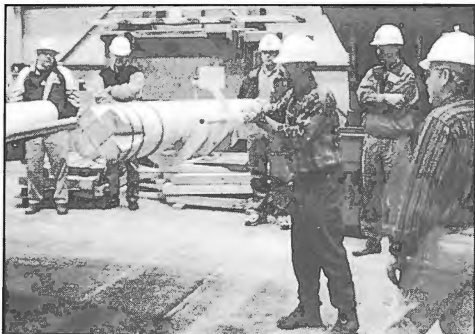
Figure 17.—Apparatus used for setting timber posts. (Photo courtesy of Strata Products USA).
