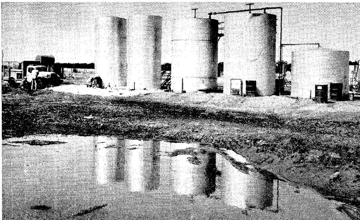
FIGURE 4. - Tank Battery Installation at the Heavy Oil Recovery Test Site.
