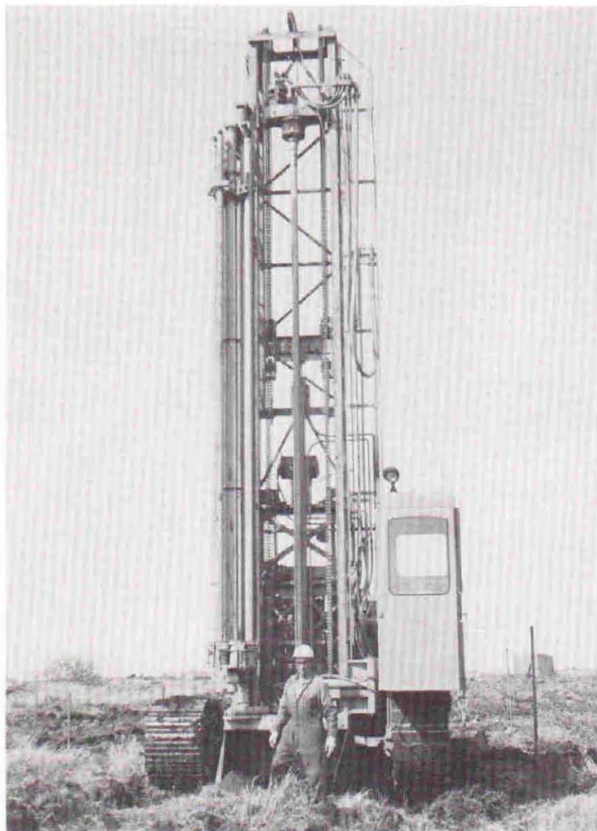
Rotary drill rig for drilling thaw holes into which heated water is pumped.
