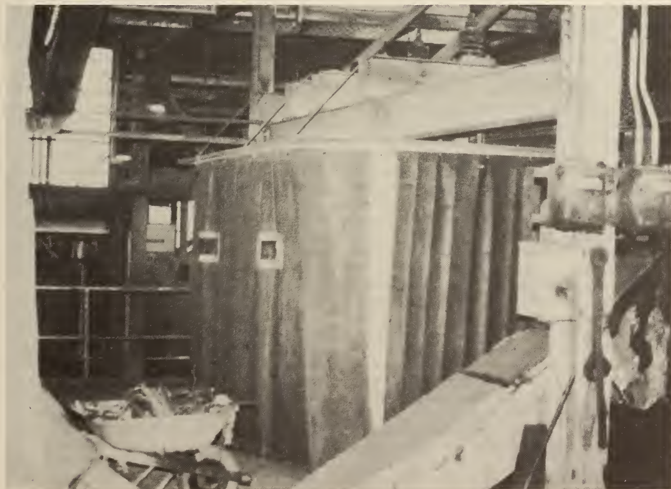
FIGURE 59. - Curtain around screening area in Georgetown coal preparation plant.
