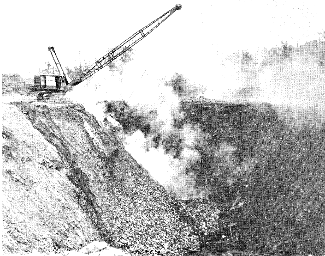
FIGURE 8. - Delaware dump during work to extinguish fire.
