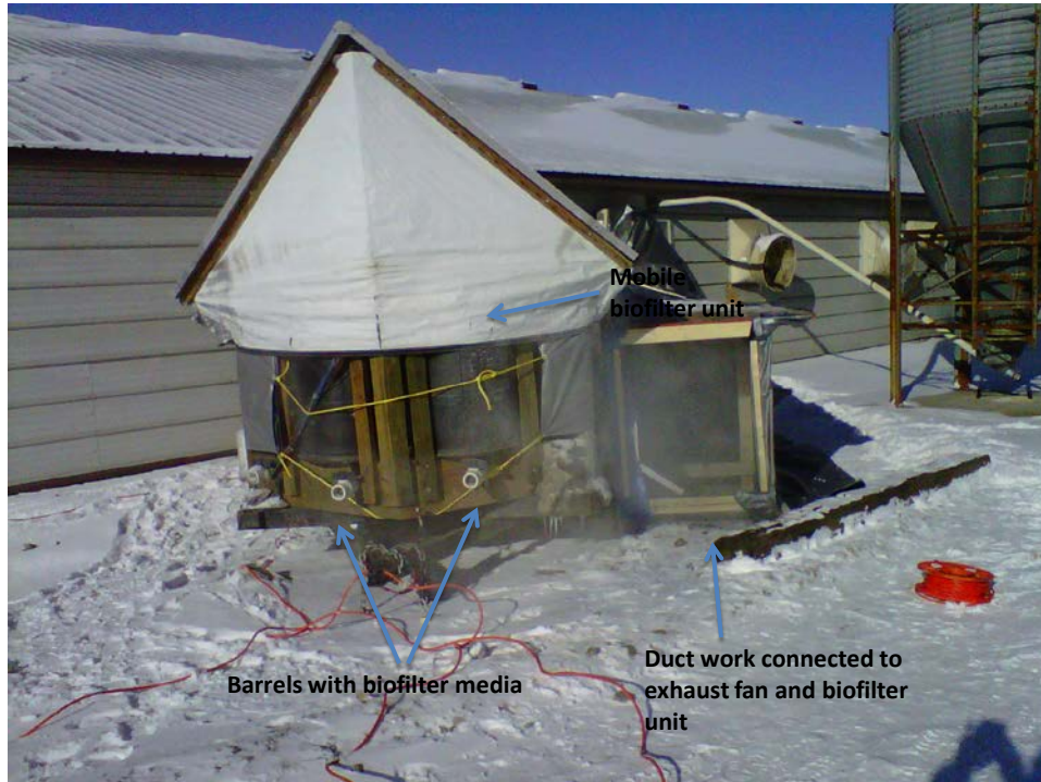
Figure 16. Biofilter mobile unit
