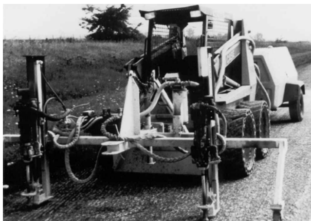
FIGURE 3 Two pneumatic drills mounted to mobile equipment being used to drill concrete pavement.
