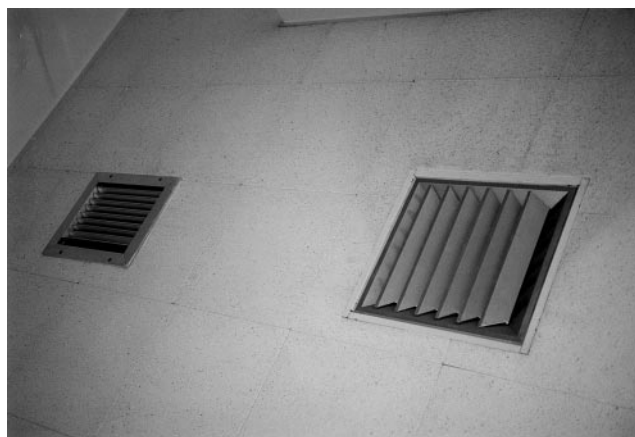
FIG. 1. An air exhaust vent in close proximity to the air intake vent in one of several offices at the public health clinic.
