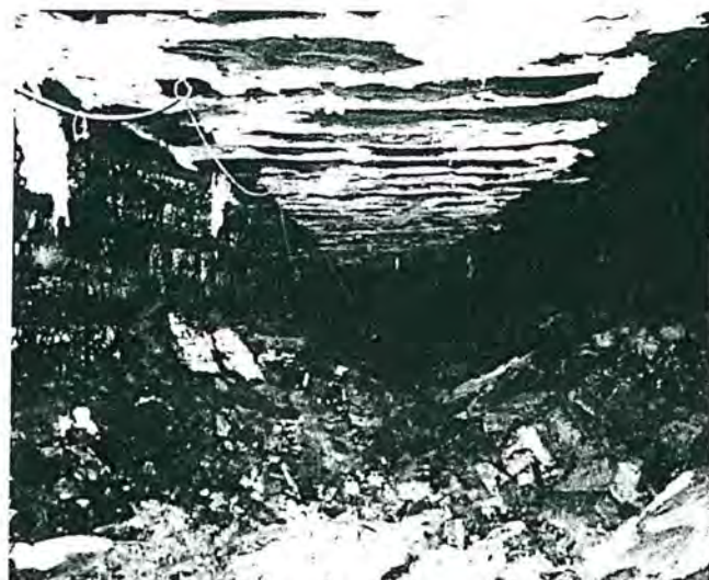
Figure 10 — Typical entry conditions after failure.
