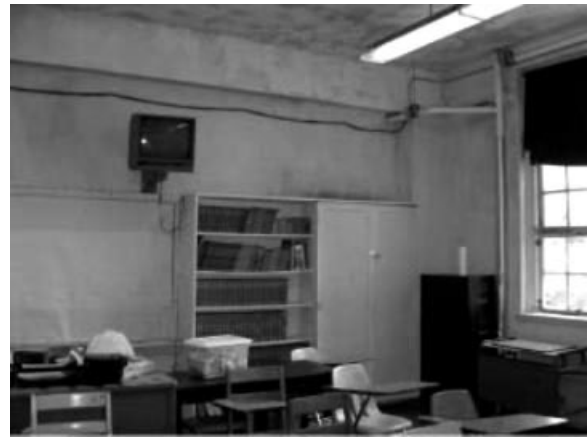
FIGURE 2. Picture of classroom wall and ceiling showing active mold growth at the water-damaged school.
