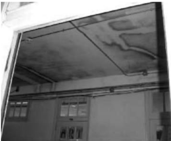
FIGURE 1. Picture of mold growing along hallway ceiling at the water-damaged school.
