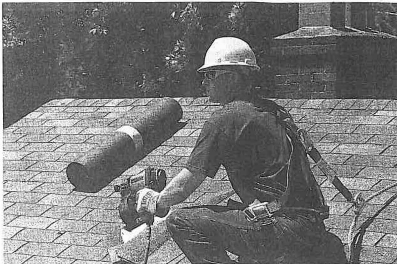
Figure 15-7. Worker wearing a full-body harness with attached lanyard properly tied off to a life line. (Photo courtesy of the Mine Safety Appliance Company.)
