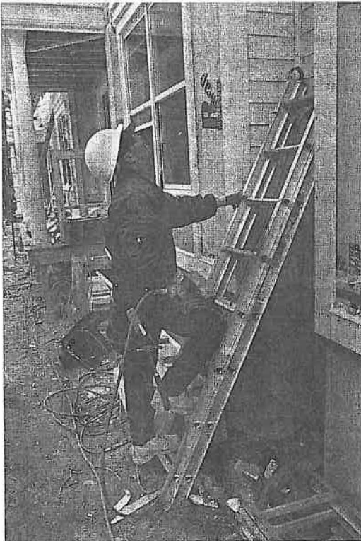
Figure 15-4. Example of poor housekeeping on a construction site. Numerous cords and debris create a potential tripping hazard for workers. (Photograph by Earl Dotter.)
