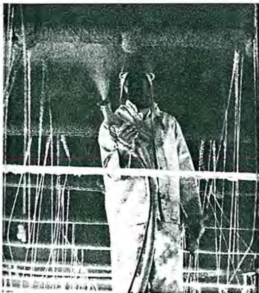
FIG. 42-5. Worker, spraying fibrous glass insulation on a building under construction, illustrates the difficulties of assessing and controlling construction-site hazards. (Photograph by Ken Light.)
