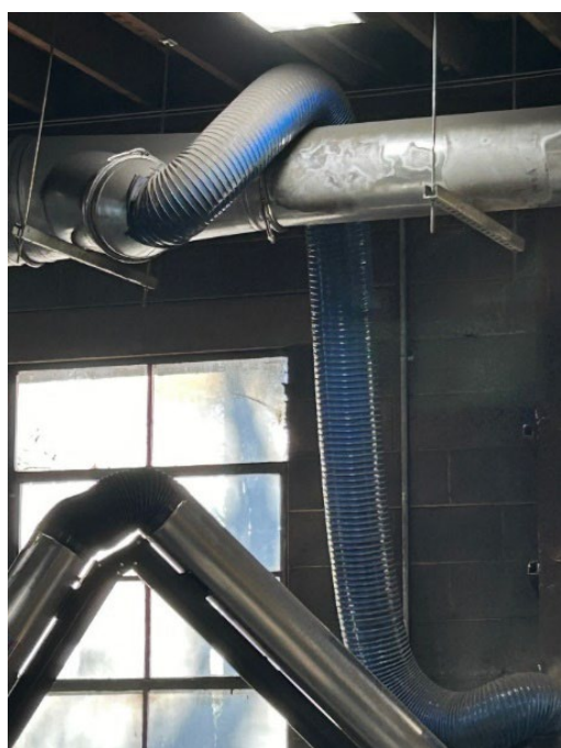
Figure B11. Flexible ductwork. Photo by NIOSH.
