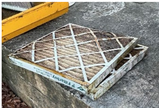
Figure B9. Dirty pre-filter. Photo by NIOSH.
