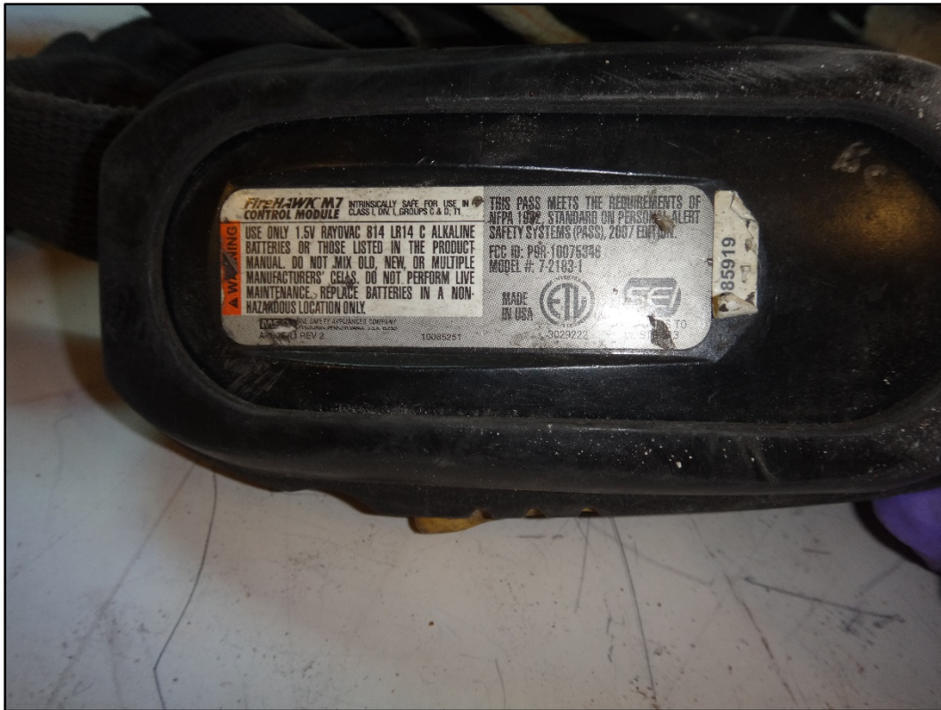
Figure 21: Back of PASS console, SEI label
