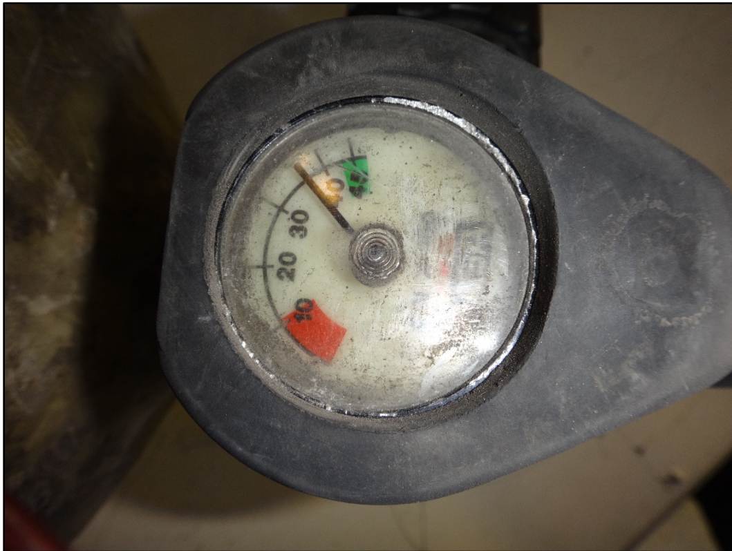
Figure 23: Gauge on cylinder connection
