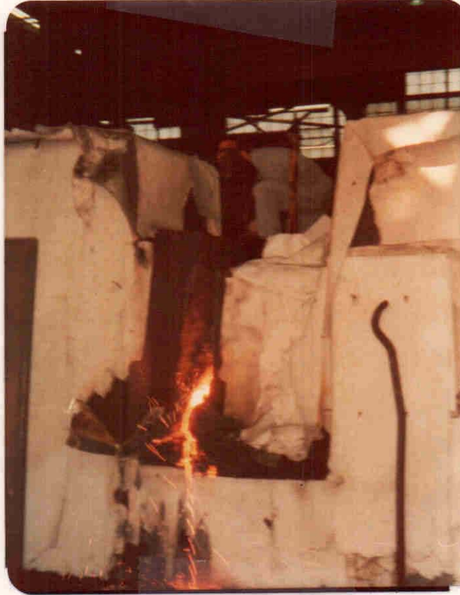
Preparing a cracked machine base for arc welding repairs. (PLANT MAINTENANCE ACTIVITY)
