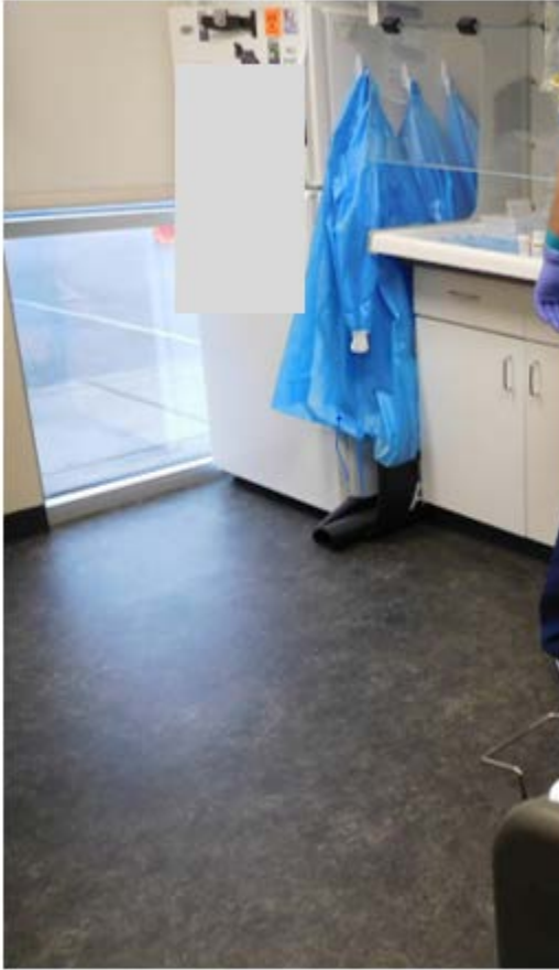
Figure 9. Floor in front of BSC in chemotherapy preparation and administration area. Wipe sample collected from wet spot on floor. (Photo credit: NIOSH)
