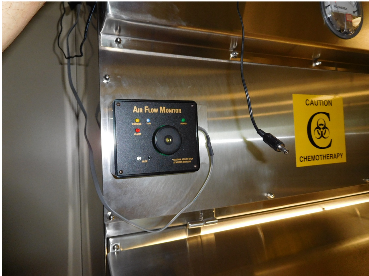
Figure 14. BSC's air flow monitor (Photo Credit: NIOSH)
