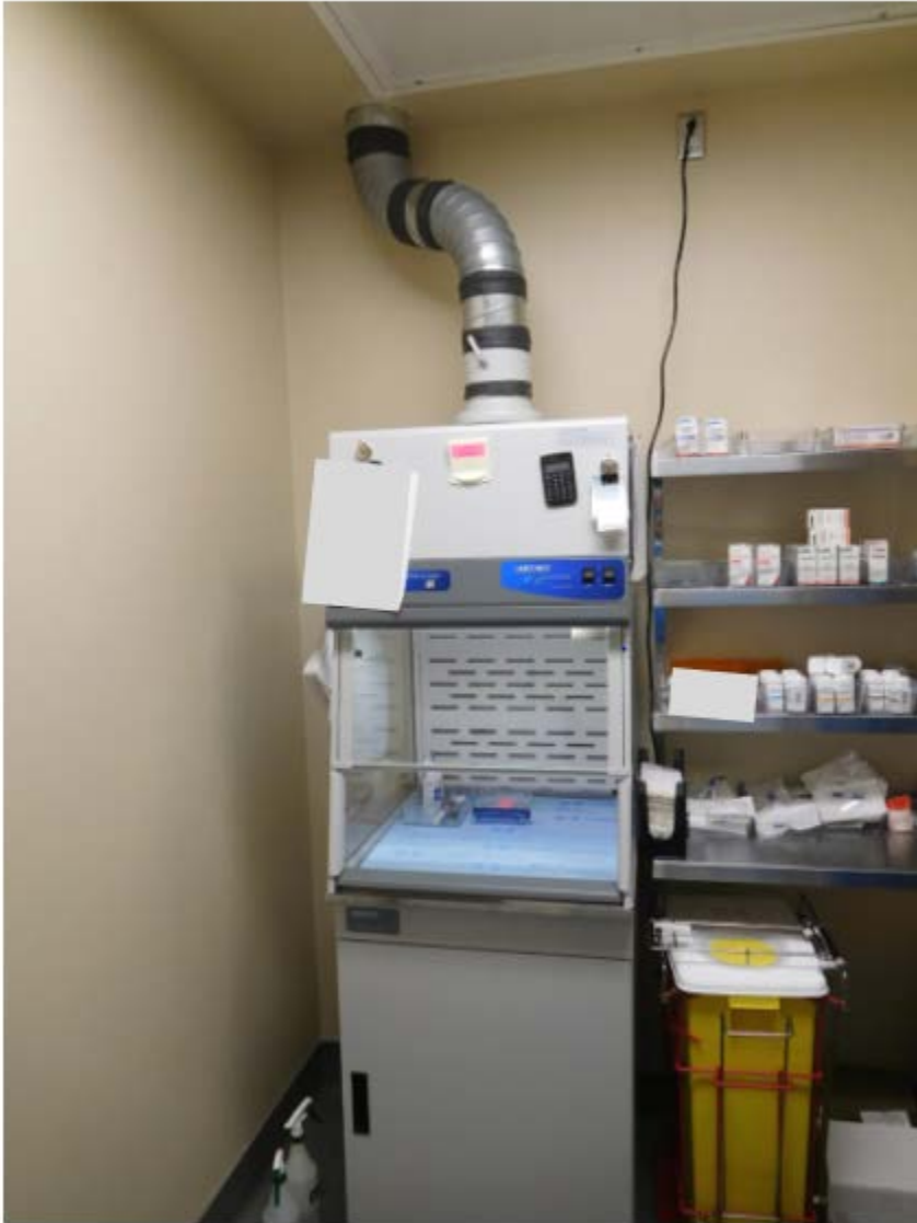
Figure 4. Oncology Department's buffer room with BSC (Photo Credit: NIOSH)
