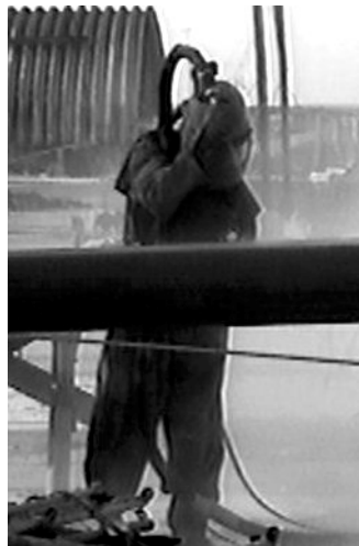
Figure 5. Abrasive Blaster Blasting Material Above Waist Height
