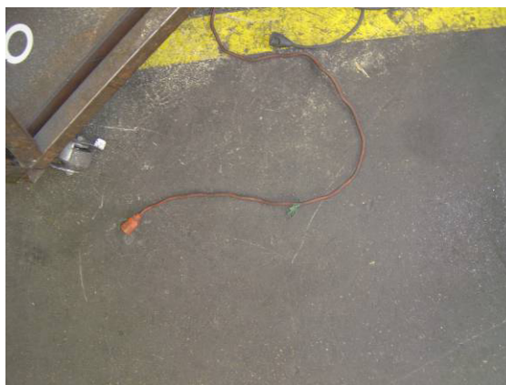
Figure 7. Damaged extension cord
