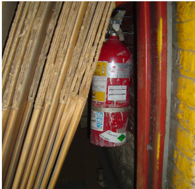
Figure 6. Fire extinguisher blocked and hidden by boxes.
