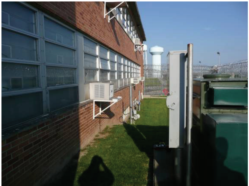
Figure 1. Transformer located within 7 feet of the exterior wall of the timekeeping office.
