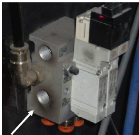
Figure 18. Exhaust ports of a solenoid valve without silencing mufflers.
