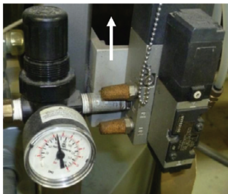
Figure 19. Mufflers on an exhaust port of a solenoid valve.
