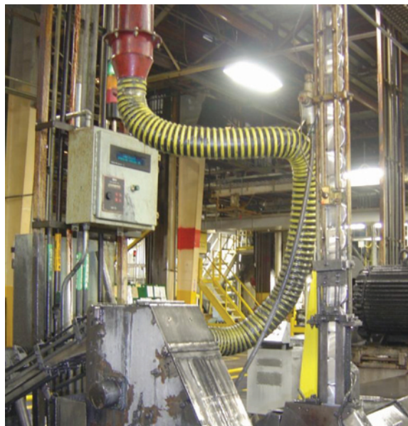
Figure 7. Flexible exhaust ventilation duct with too many bends at an ironer, which reduces effective ventilation.
