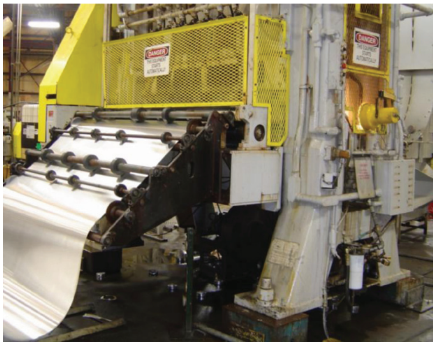
Figure 13. Large copper press, without vibration damping, mounted to the concrete floor.
