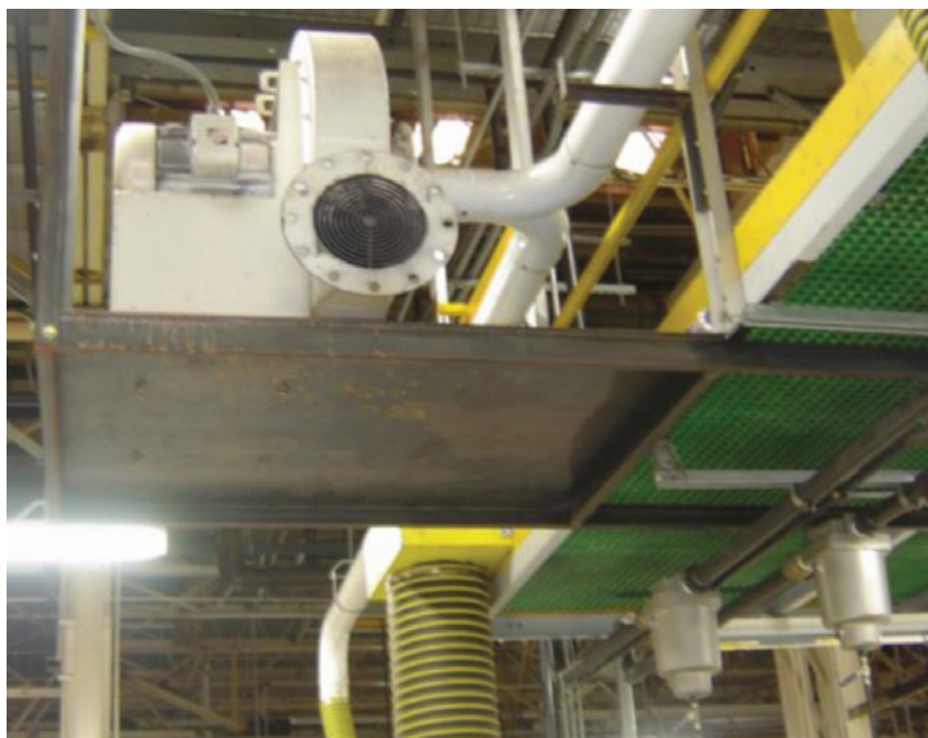
Figure 14. Motor and blower, without vibration isolation or noise enclosure, mounted directly to a metal platform above the necker line.
