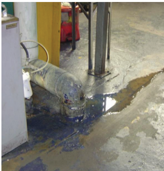
Figure 6. Water on floor near Concord printers.
