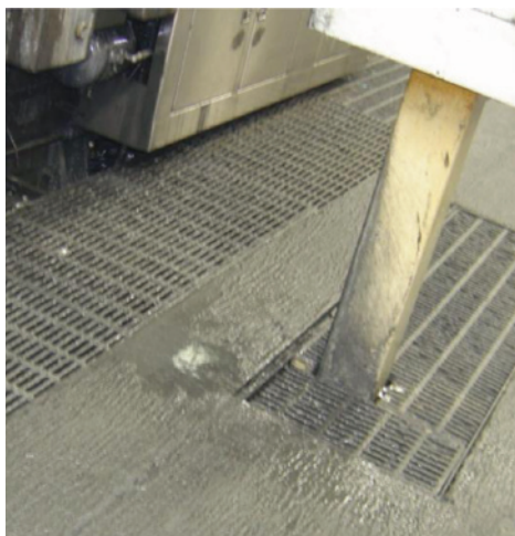
Figure 4. Metalworking fluid on floor in ironer area.
