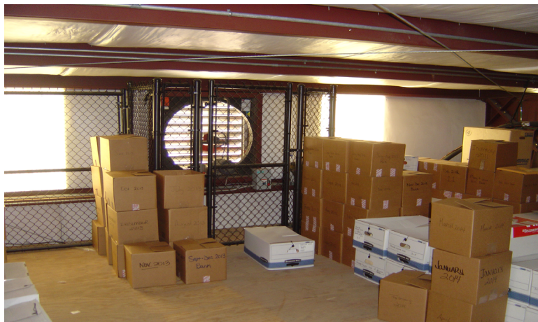
Figure 4. Boxes stacked around a warehouse exhaust fan. Photo by NIOSH.
