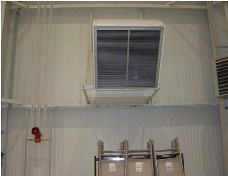
Figure 2. Photo of supply fan shroud oriented at a 30 degree down angle. Photo by NIOSH.
