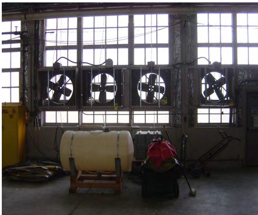
Figure 4. Photo of window-mounted wall exhaust fans inside a restoration hangar. Photo by NIOSH.
