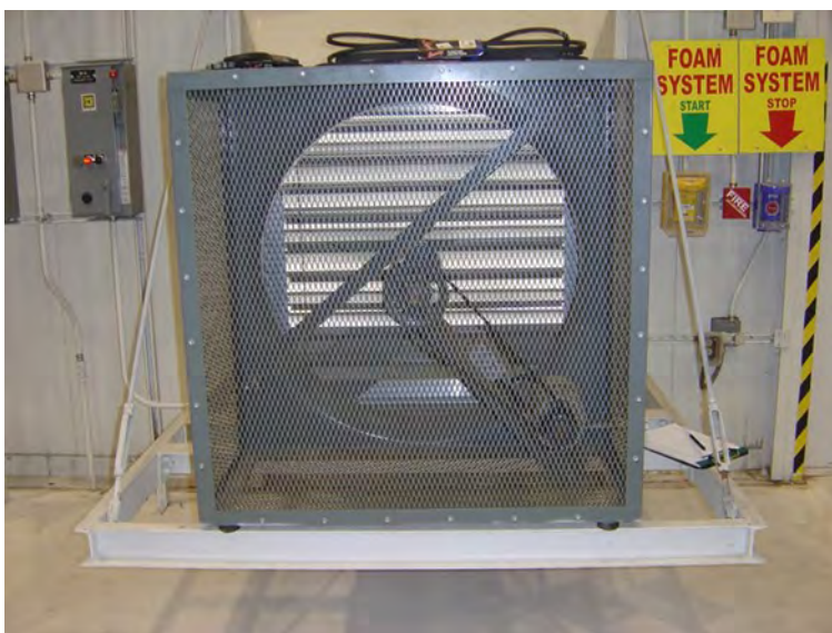
Figure 3. Photo of an exhaust fan extending straight through the exterior wall. Photo by NIOSH.
