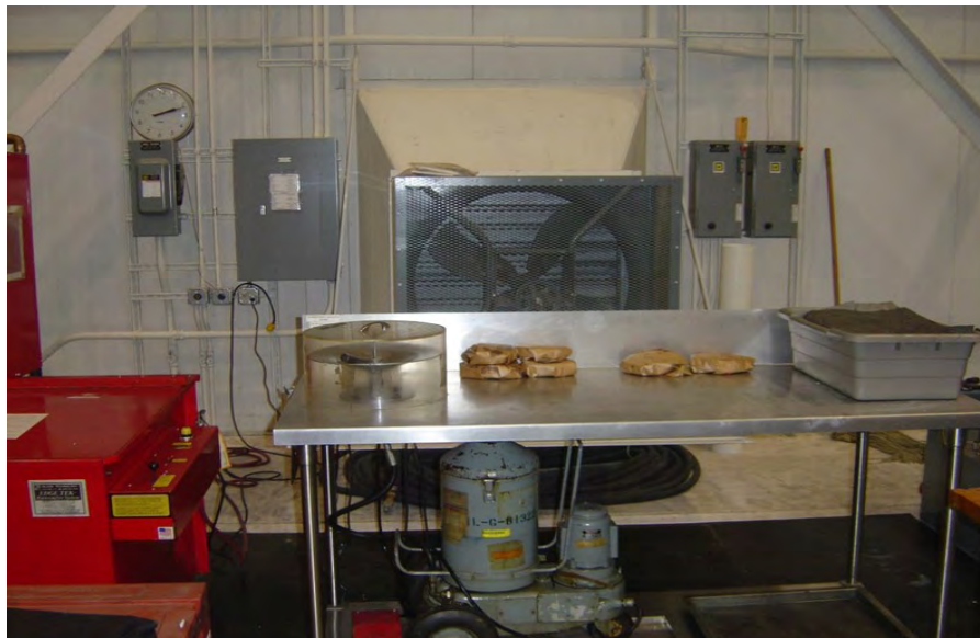
Figure 10. Photo of table and equipment blocking exhaust fan outlet. Photo by NIOSH.
