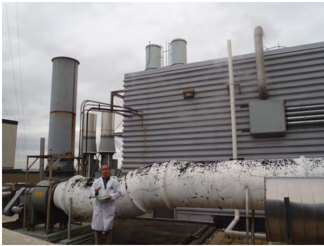
Figure 3. Rooftop penthouse exhaust pipe (shown in the upper right corner of the figure), which was located adjacent to NRC-AHU-5. Prevailing winds carried exhaust from the pipe toward the NRC-AHU-5 supply air intake. Photo by NIOSH.
