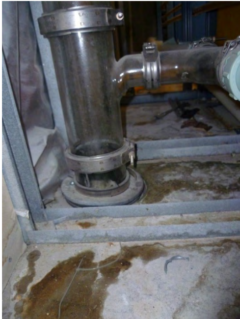
Figure 2. Photo of gap between utility drain pipe under laboratory cabinet and floor provided unplanned pathway for movement of air from floor below. Photo by NIOSH.
