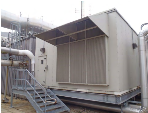
Figure 4. Photo of a supply air intake for rooftop air handling unit, NC-AHU-5, where building exhaust air was observed being captured by the intake. Photo by NIOSH.
